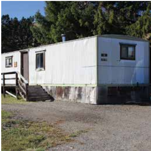
ABOVE Decades-old mobile homes serve as summer staff housing at Mammoth Hot Springs in Yellowstone National Park, an example of the hidden, nonpublic aspect of the maintenance backlog.
