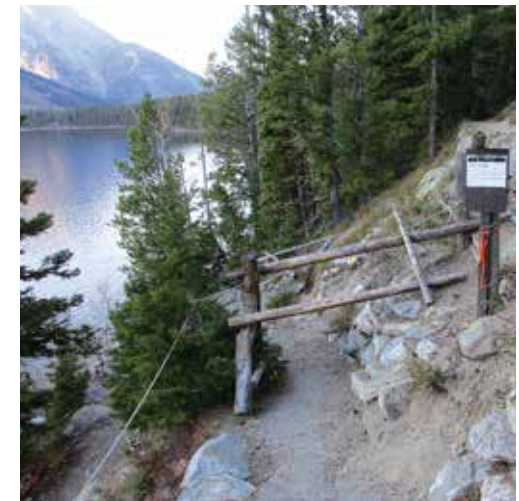
ABOVE This trail at Jenny Lake in Grand Teton National Park has been eroded by heavy use and rough weather to the point where it has been closed for safety reasons.
