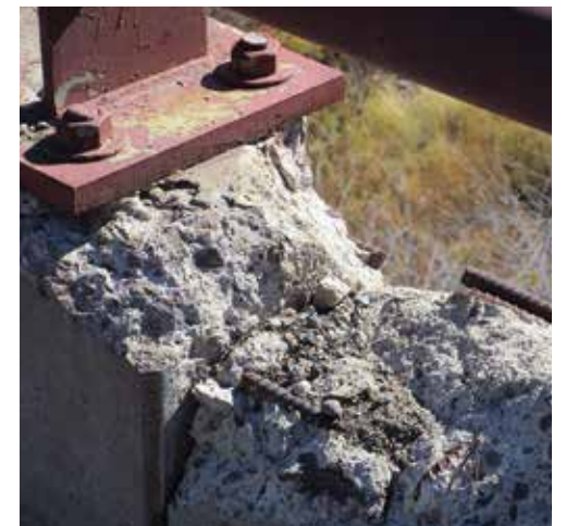
ABOVE Compromised reinforced concrete on the Yellowstone River bridge exposes rebar, which accelerates the decay of the aggregate matrix.
